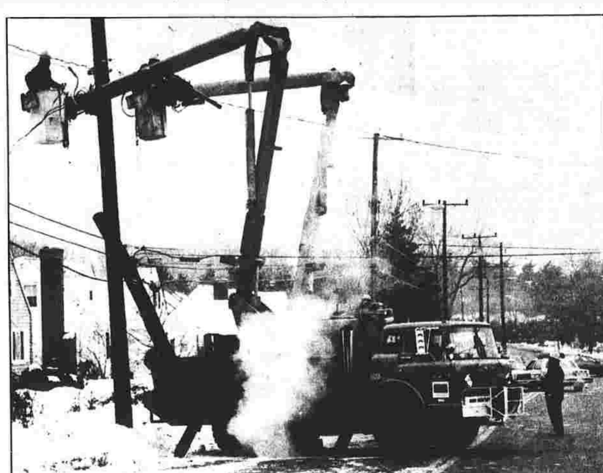
RESTORING POWER - Northeast Utilities crews repair a pole and fallen power lines early today on West Middle Turnpike just west of Adams Street. A car hit the pole Thursday night near the intersection of West Middle Turnpike and Hendee Road. The accident caused a loss of power for more than 2,700 customers in the north end of town.
